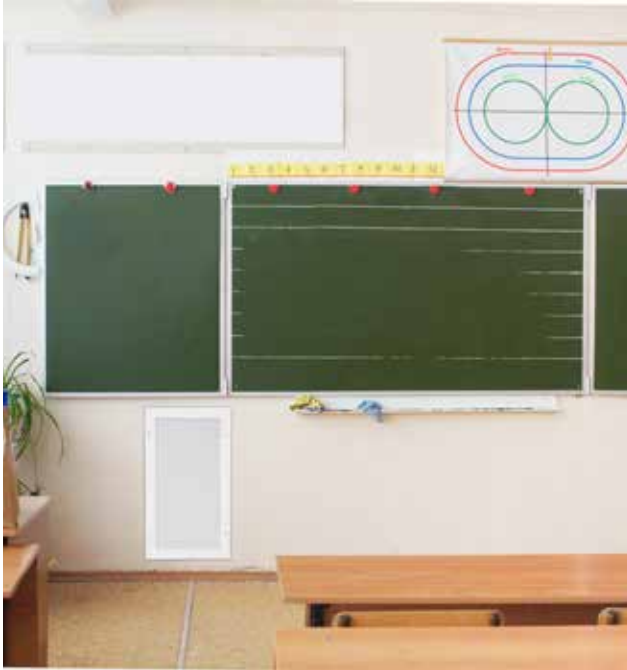
Example of an internal wall mounted diffuser.
