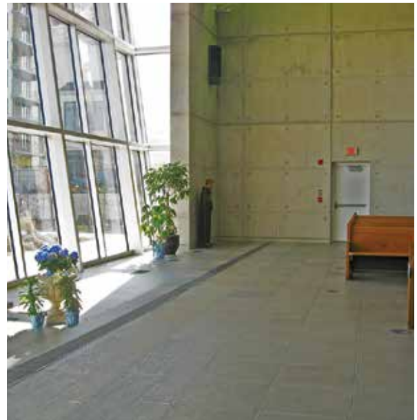
Example of a floor mounted diffuser.
