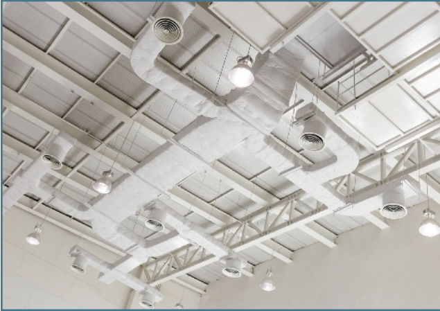
PHOTO 3. Round diffusers installed in an open ceiling. tavizta/Shutterstock
